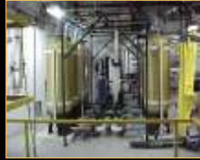
Large DI Water System
