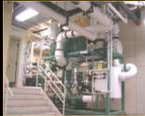
Steam-Hot Water Exchange Unit (Packaged)
