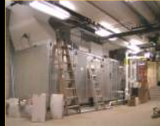
AHU Unit for Office/ Administration Areas
